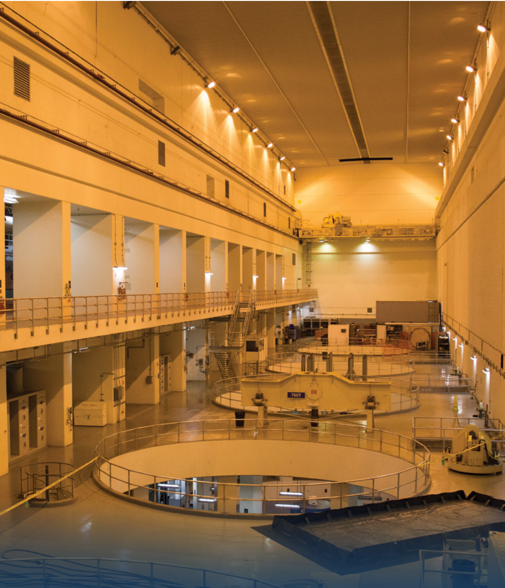
Dominion Energy's Bath County Pump Storage facility in Virginia
